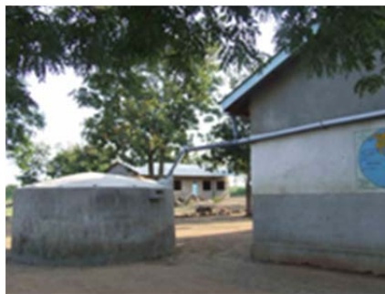
Existing roof top rain water harvesting facility
