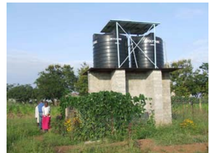
Existing production borehole with solar powered pump
