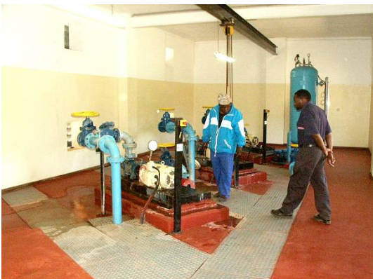
Pumping station at Quthing water treatment plant
